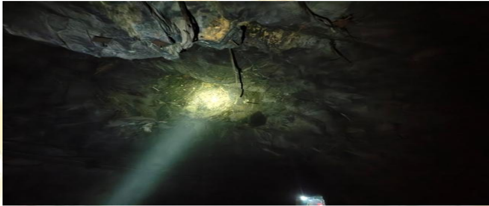
Fig. 5: Wedge failure observed at 89mRL decline drive.
