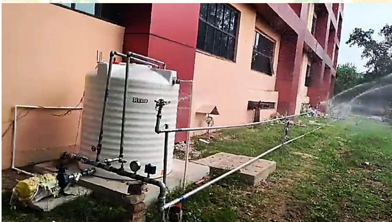
Fig. 1: View of the installed automatic wireless sprinkling system
